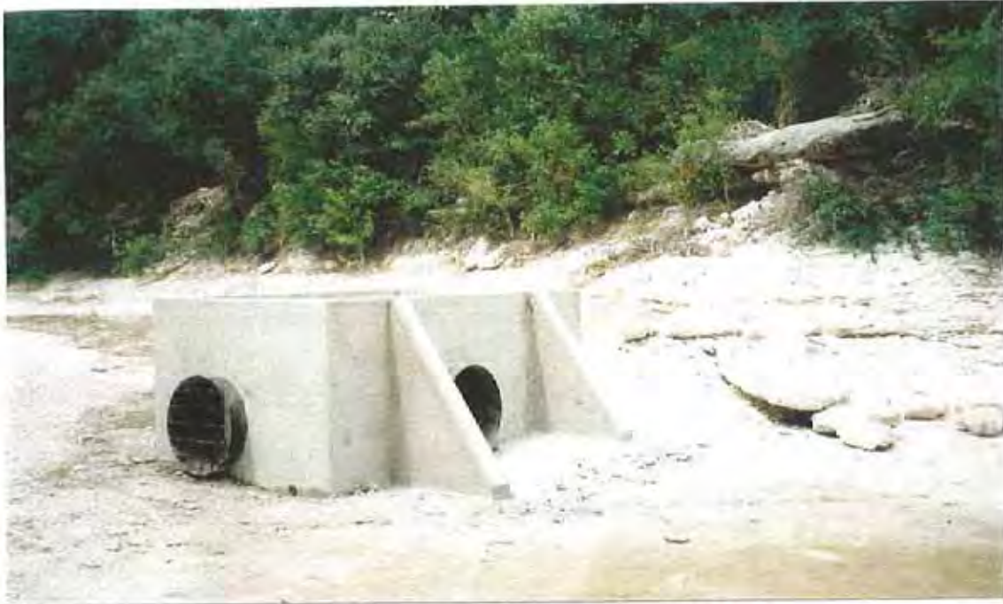
Antioch Cave BMP as installed in 1997.
