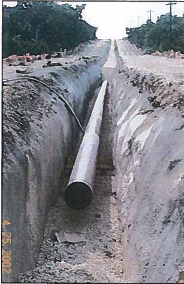
Figure 9. Longhorn Pipeline with gunite lining of trench. Photo courtesy of Barton Springs/Edwards Aquifer Conservation District.
