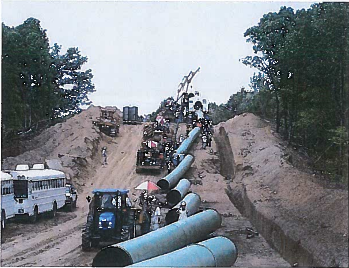
Figure 2: Photo of construction of a representative 42-inch pipeline in a 125-foot wide easement.
