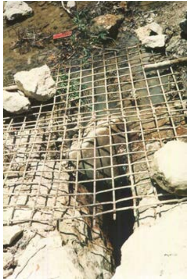
Fig. 2 Photograph ca. 1996 showing recharge and the entrance to Antioch Cave before the BMP was constructed. The debris over the entrance and also sedimentation within the cave decrease the amount of recharge entering the cave (Photograph from Fieseler 1998)
