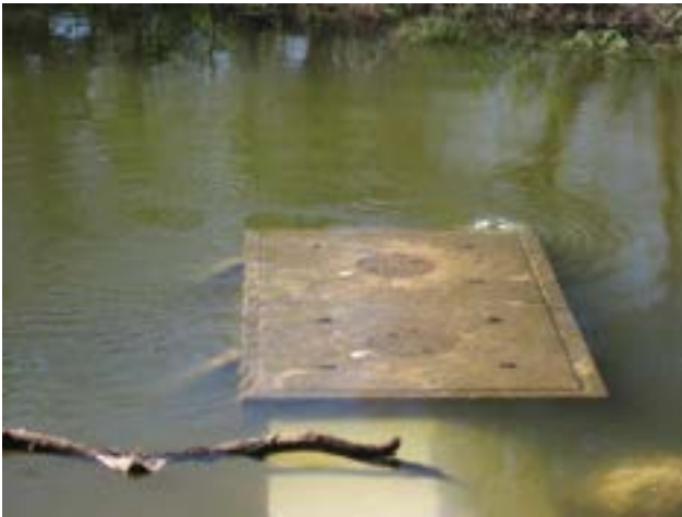
Fig. 11 Photograph of the top of the BMP about 8 h past the peak storm pulse on October 27, 2009, with a whirlpool near the corner of the vault due to water entering the original valve
