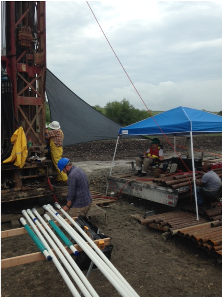
The monitor well is 1,095 feet deep and goes from the Taylor Clay at the surface through the Edwards formations into the Upper Glen Rose formation. It was constructed to isolate 18 individual zones
